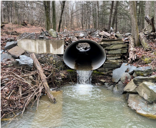
Before: Large scour pools, undersized culverts, ditch scouring and large deposits of sediment from flood damage.
